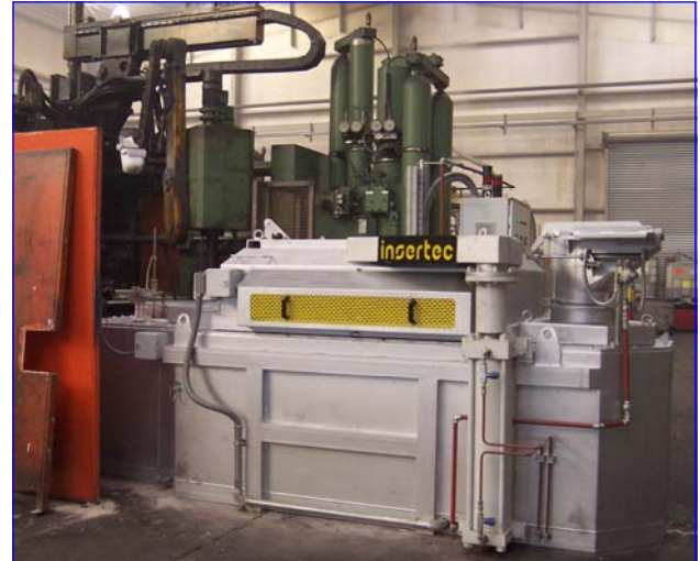
RMAE Holding Furnace next to High Pressure Die casting Machine.
