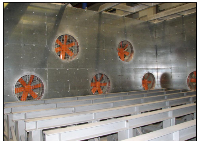
Forced Air Cooling Chamber.
