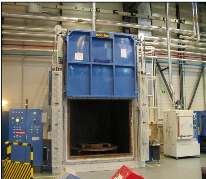
Chamber type Recirculation Furnaces.
