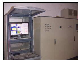
Electric Control Panel with computer system.
