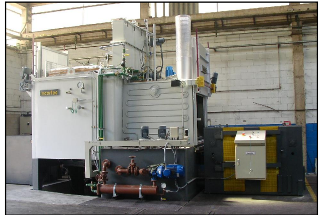
General view of Transfer Furnace provided with charging and discharging machines.
