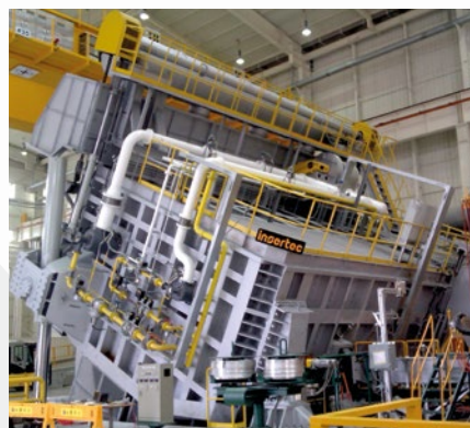
\ Tilting reverb furnace
