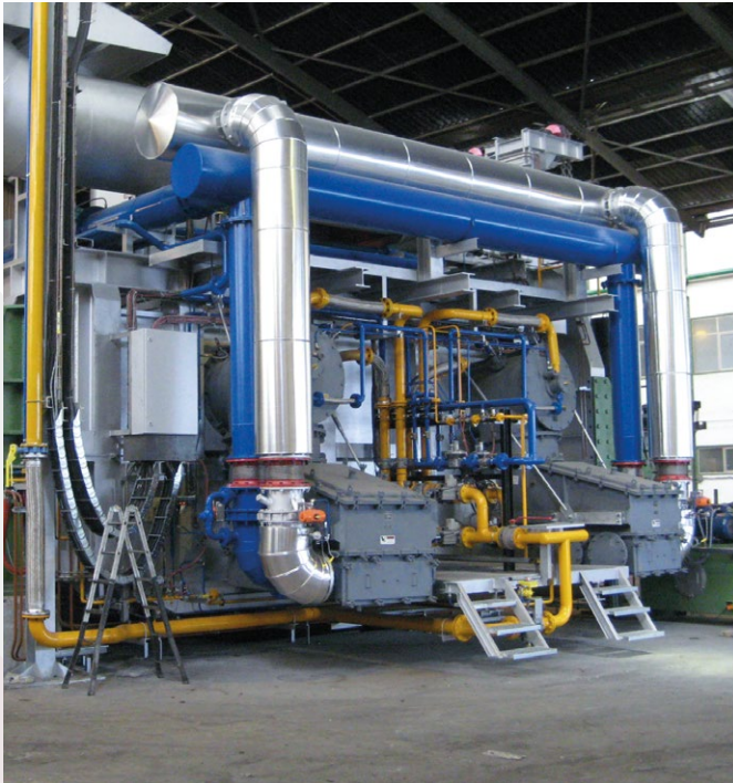
\ Regenerative burners on melting reverb
