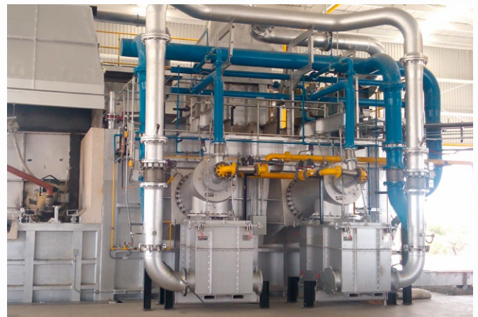
\ Sidwell melter 65 Ton with regenerative burners.
