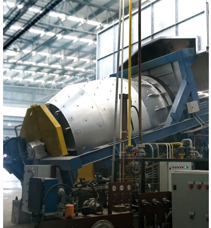
\ Tilting rotary furnace
